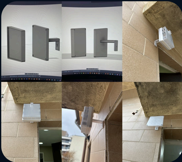
EDS station development and installed enclosure. These are station-context images, not eclipse photographs.
